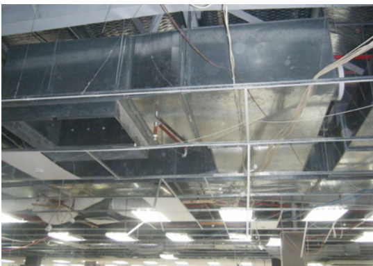
Figure 64: Lack of suspension points and service clearance.
