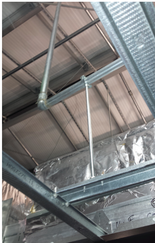
Figure 66: Sprinkler system supported from ceiling componentry rather than suspended from the building structure.
