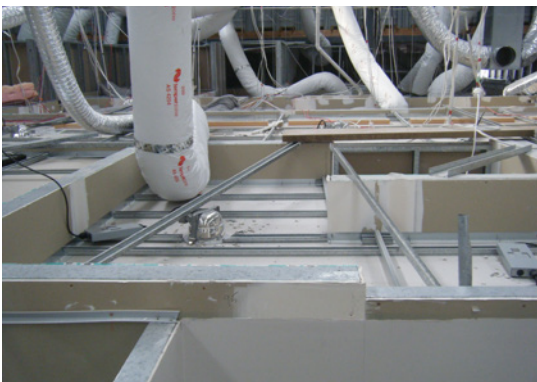
Figure 65: Unbraced partitions and service ducts.
