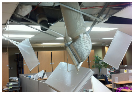
Damage caused by unrestrained ducting.
